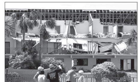
Class of 1955: Hurricane Irma damage, St. Augustine Beach
